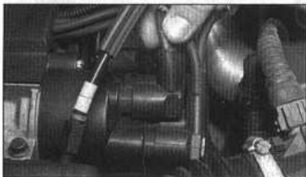
A Check that the HT leads are securely connected to the distributor and that the cap is clean and properly fitted
